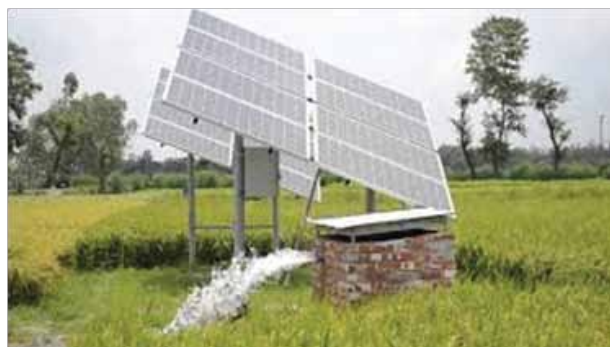
Finance in Solar pump
