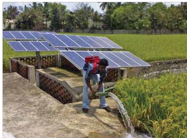
Investment in Solar Pump
