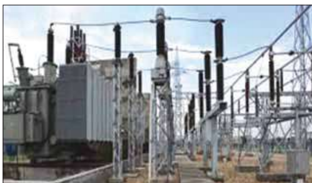
Orion Power Plant
